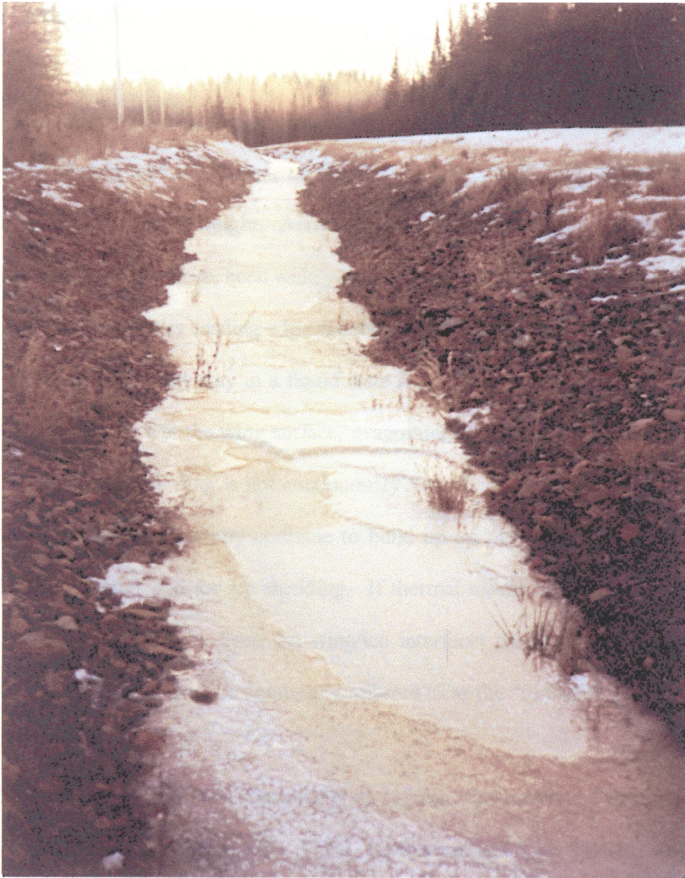
Figure 2.1 Aufeis formation in a drainage ditch.
